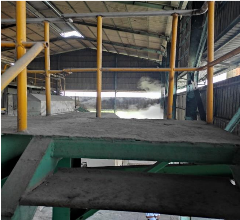
Photo 9: Platform of the stairs (PT BAS) lacking appropriate toe boards
