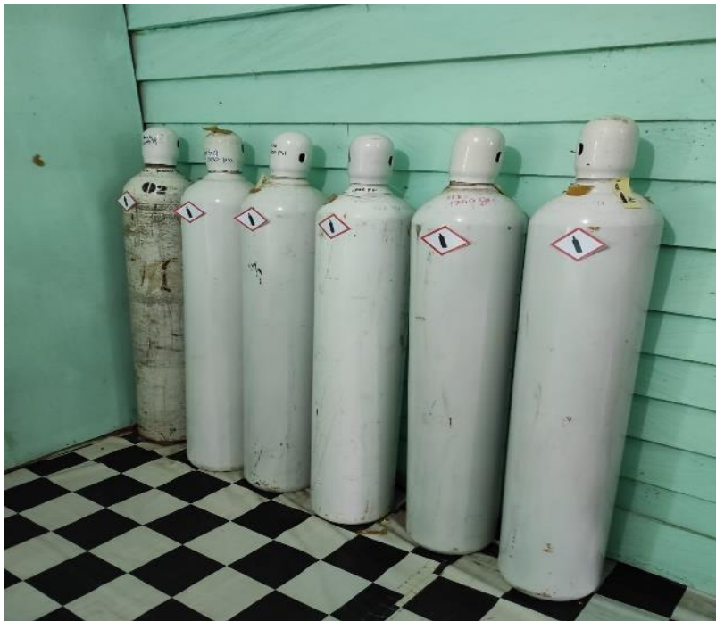
Photo 8: Cylinders of Oxygen at Clinic (PT BAS) lacking labelling, safety chain or appropriate signage
