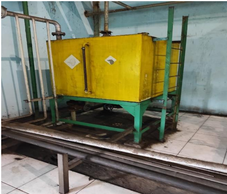
Photo 10: Diesel fuel storage tank, lacking in appropriate bunding and signage (PT BAS)
