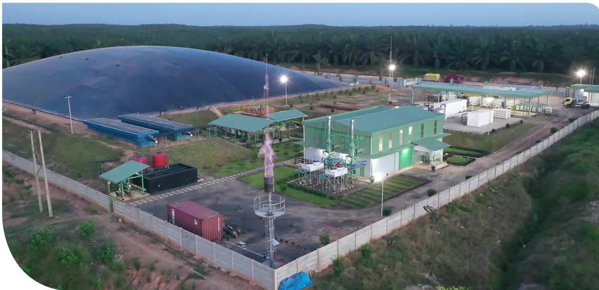
Fasilitas Bio-CNG DSNG di Muara Wahau, Kalimantan Timur DSNG Bio-CNG's facility in Muara Wahau, East Kalimantan
