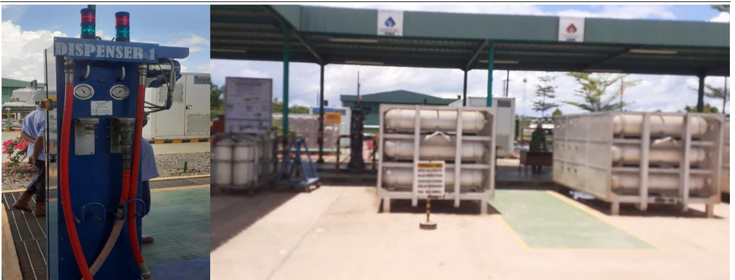
Exhibit 14. Bio-CNG dispenser (LHS) and deployable Bio-CNG tanks ready to distributed (RHS)
